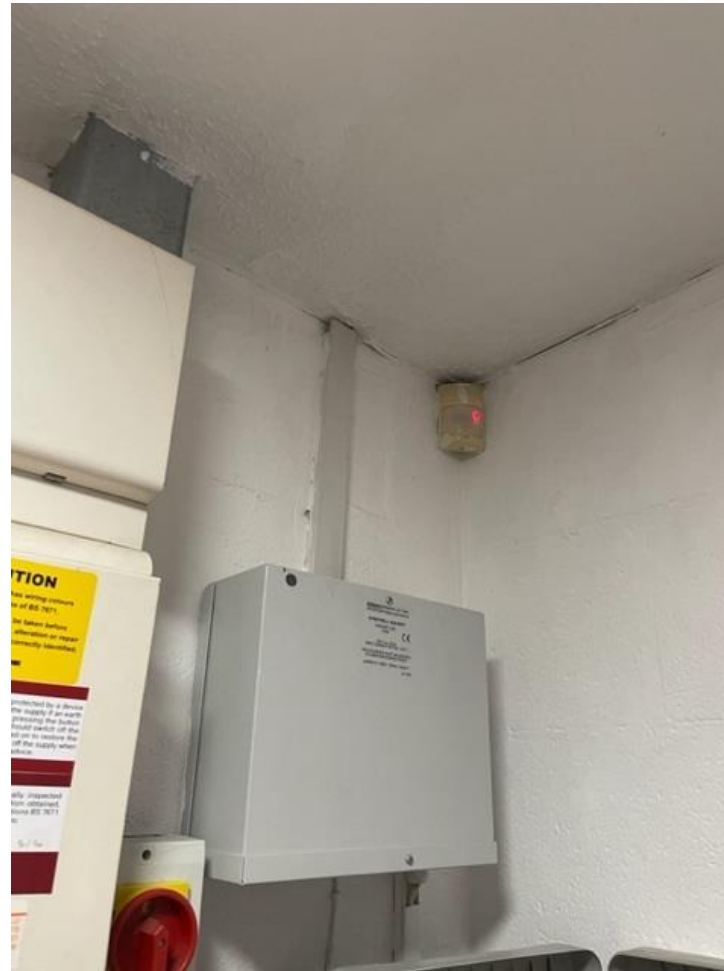
Photograph 2: Penetrations through ceiling in electrical cupboard
